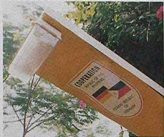
Community streetlight in Sablayan, Mindoro. A 53 Wp panel operates 11W compact fluorescent lights all night. The simple design combines all electronics in the sealed light casing.
