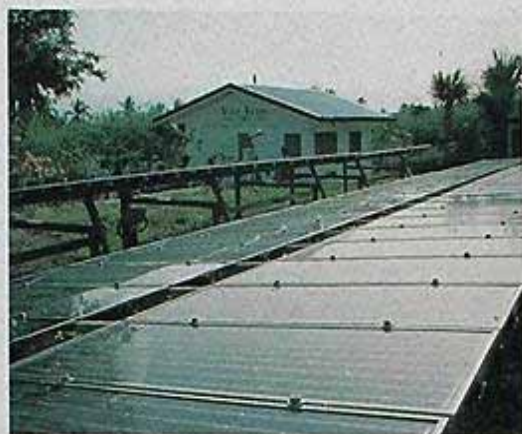
Central PV Plant, San Agapito, Isla Verde. 6000 Wp serve 220 VAC to 28 households via a 1 km grid. Later improvements rendered the same service level with a 2000Wp generator.
